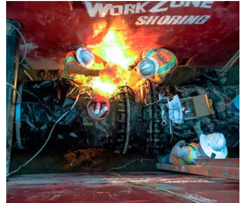
Joint bond welding on a 36" ductile iron pipe at 22nd Street and Alvernon Way. Pictured above is Nick Zedaker, Andrew Joyal, and Angel Perez.
